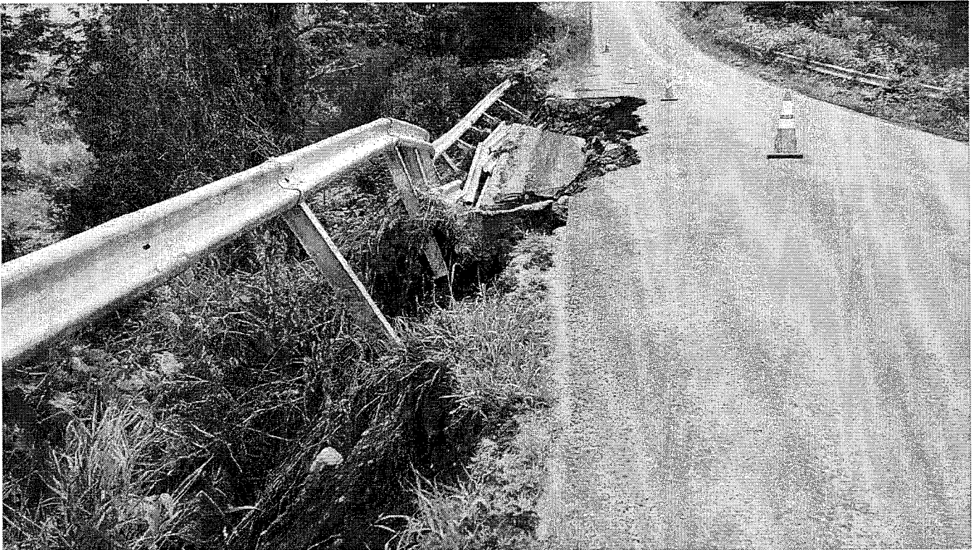
Damages on Maxwell Road in the Town of Marshall, facing east. The damages are on the downstream side of the road.
