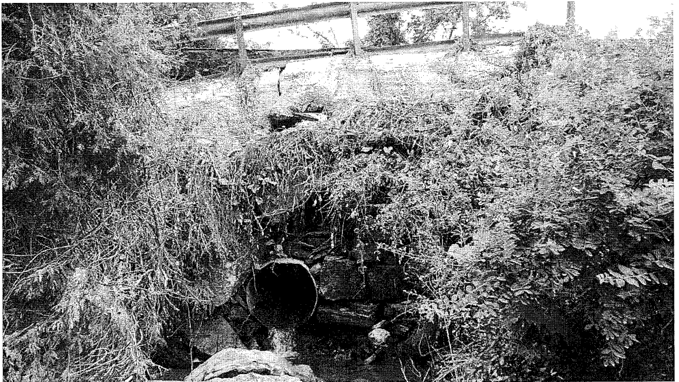
Existing perched 3' diameter corrugated culvert to be replaced by pipe arch with baffles. New culvert will be 60 feet long instead of 50 feet long. The downstream invert will be placed at the elevation of the bed.
