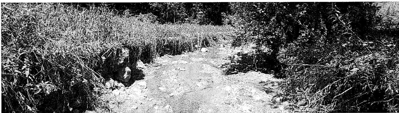
Approximately 500 feet downstream of the existing culvert facing downstream. Channel has scoured to clay and banks are erosive.
