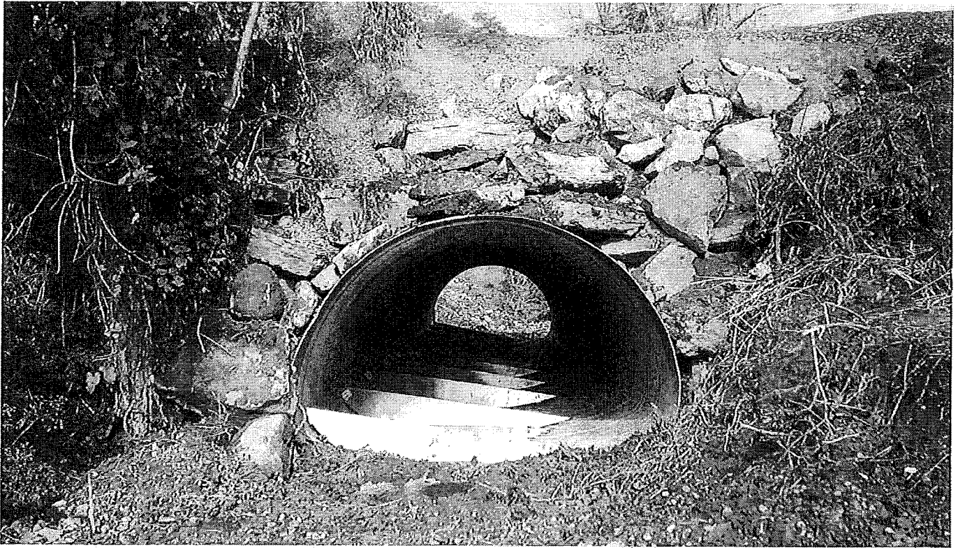
Facing downstream at the upstream extent of the new 143" span culvert with baffles. Baffles are spaced at 6' intervals. Photo 10.5.17.
