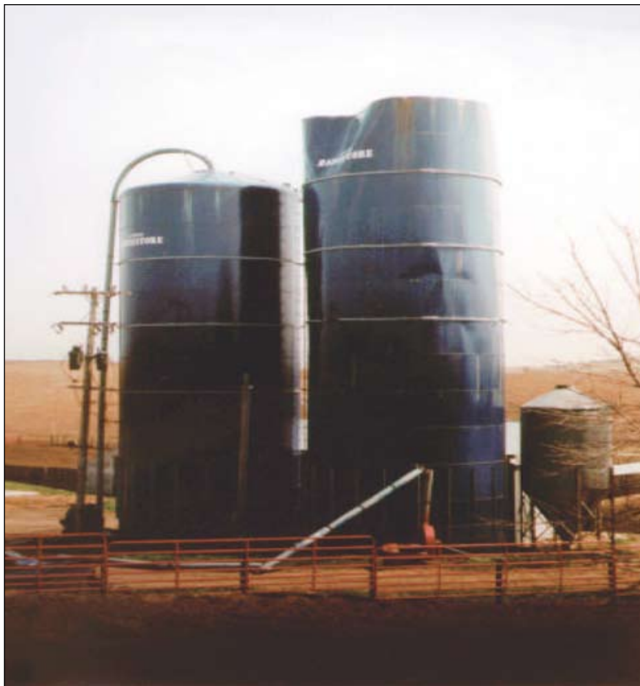
Deformity of silo shell due to explosion
