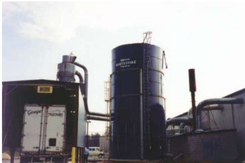
One portion of the roof traveled approximately 400 feet to the right.
