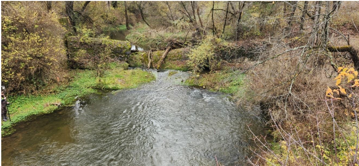
Figure 8-2. Madison Power Company Dam upstream of Solsville Road, Town of Madison, NY.
