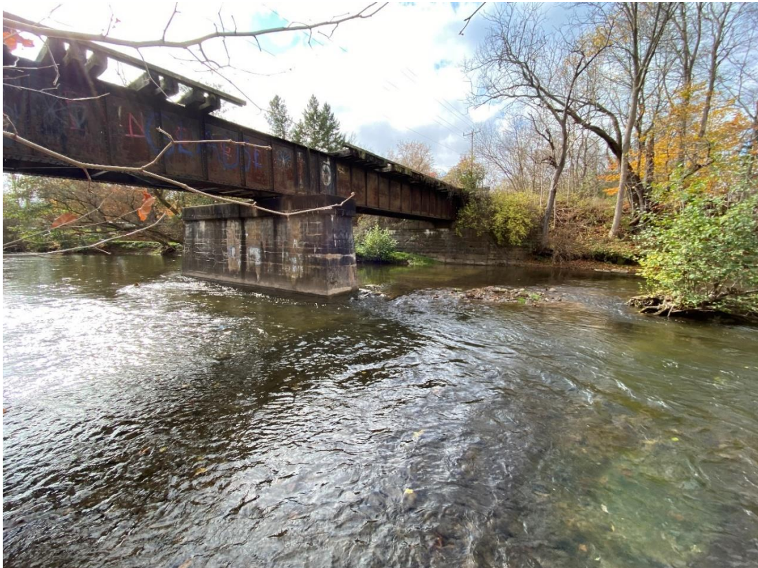
Figure 8-28. Existing conditions of the abandoned railroad bridge in Village of Clarks Mills, Kirkland, NY.
