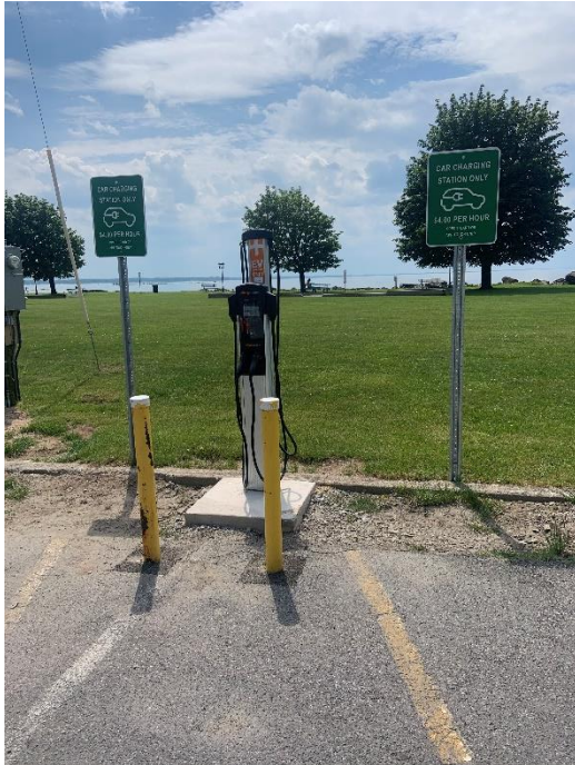
FIGURE 5.14: Sylvan Beach Electric Vehicle Charging Stations
