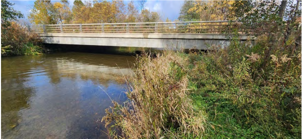
Figure 8-22. Upstream view of Oriskany Creek under the NY-5 Bridge in the Town of Marshall, NY.
