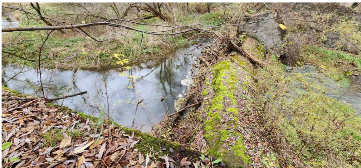
Figure 8-1. Woody debris collection upstream of the Madison Power Company Dam, Town of Madison, NY.
