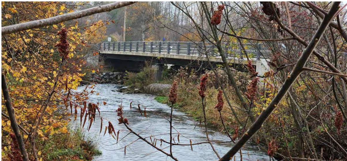
Figure 8-17. Upstream view of Oriskany Creek under the NY-315 Bridge in the Town of Marshall, NY.
