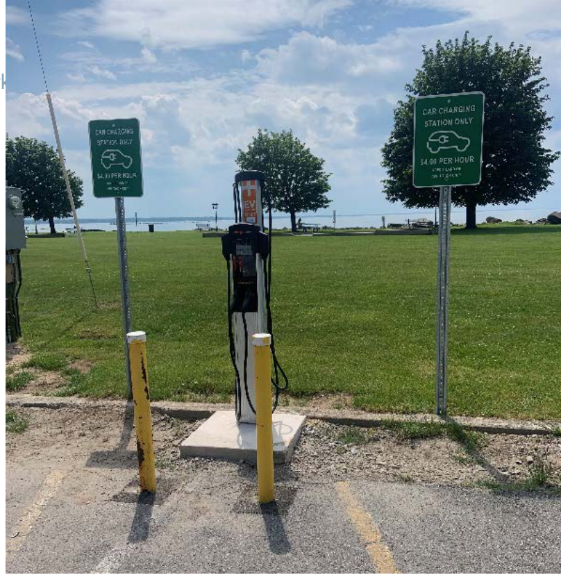
FIGURE 5.14: Sylvan Beach Electric Vehicle Charging Stations
